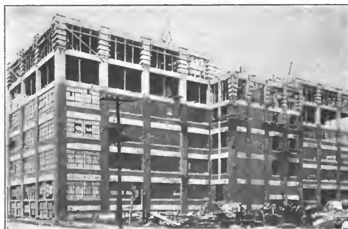
New factory of Hyatt Roller Bearing Co., Newark, N. J., to provide for the increased demands for its product. The new structure is 75 by 200 feet and will comprise six stories and a basement. The building is of cement and steel construction, conforming with the general plan of the others in the group. The work now has reached the top story and the machinery already is being placed on the lower floors
